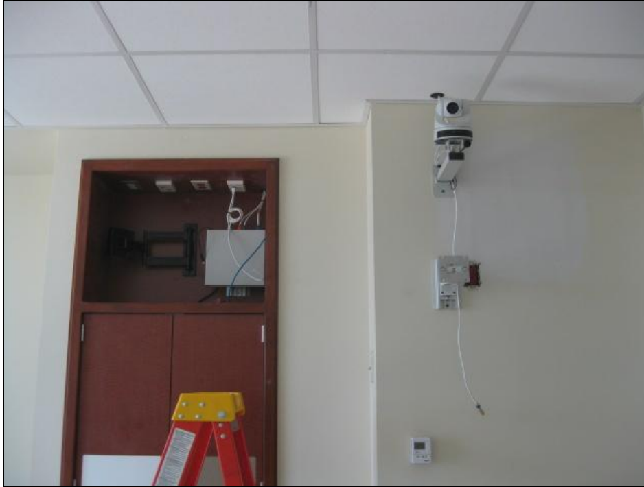
E-Care installation in ICU (4 West)
